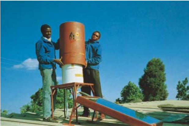
Fig.: 2: Assembly of a plant with a storage volume of 100 litres. The vertical, pressure-free storage tanks can be easily manufactured and have a very good stratification behaviour. They are filled using a float valve.
