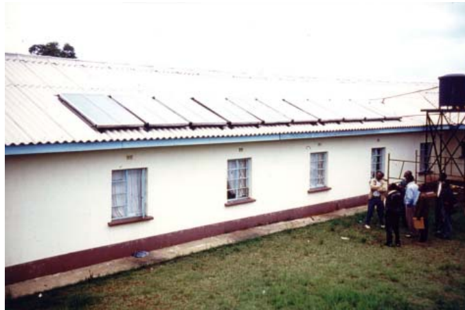
Fig.: 4: One of the plants erected at St. Johns Secondary School. The solar heating systems have a collector area of 20m 2 and a hot water storage tank with a capacity of 1,200 litres.
